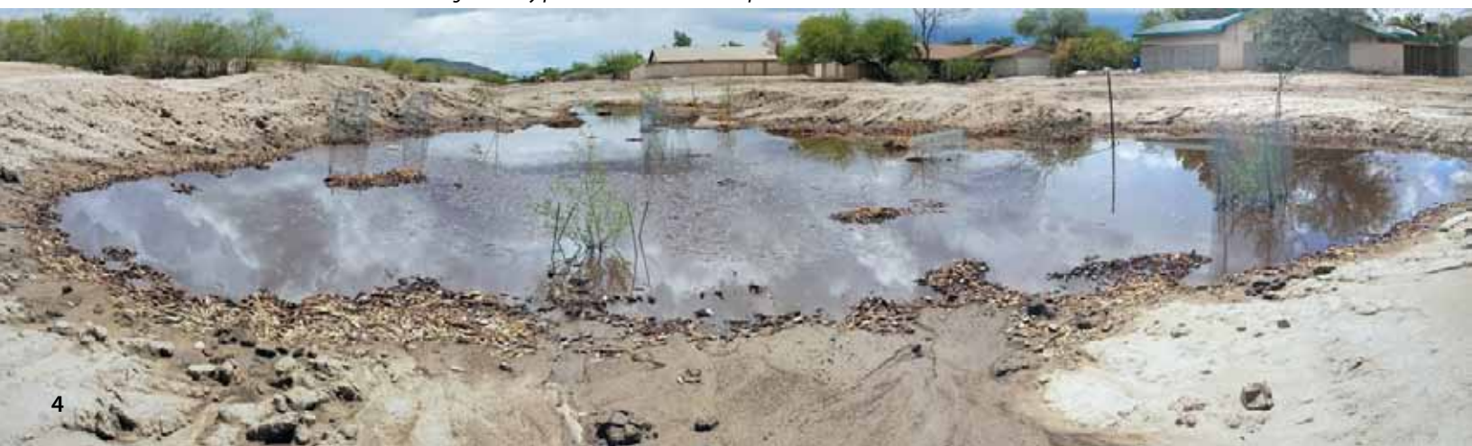
Massive basins collect monsoon rains to irrigate newly planted native velvet mesquite and desert willow trees near the Santa Cruz River.
